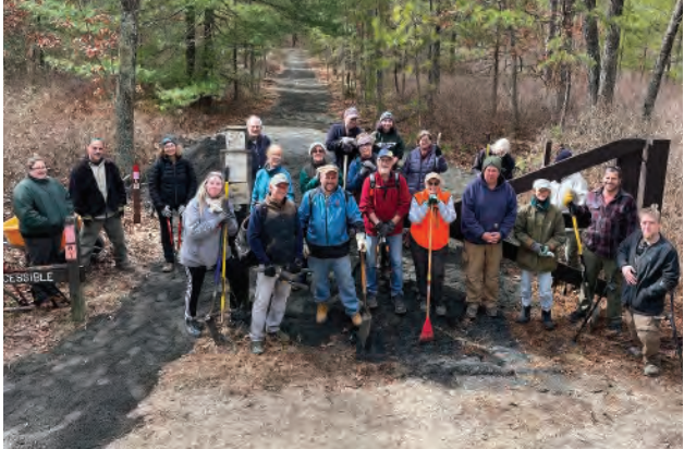
In 2023 Access Nature volunteers from the Outdoors Club of South Jersey helped Brendan Bryne State Forest improve their ADA Cranberry Trail. Volunteers helped spread stone dust on the trail to provide a more stable surface making the trail easier to use for people with mobility issues.
