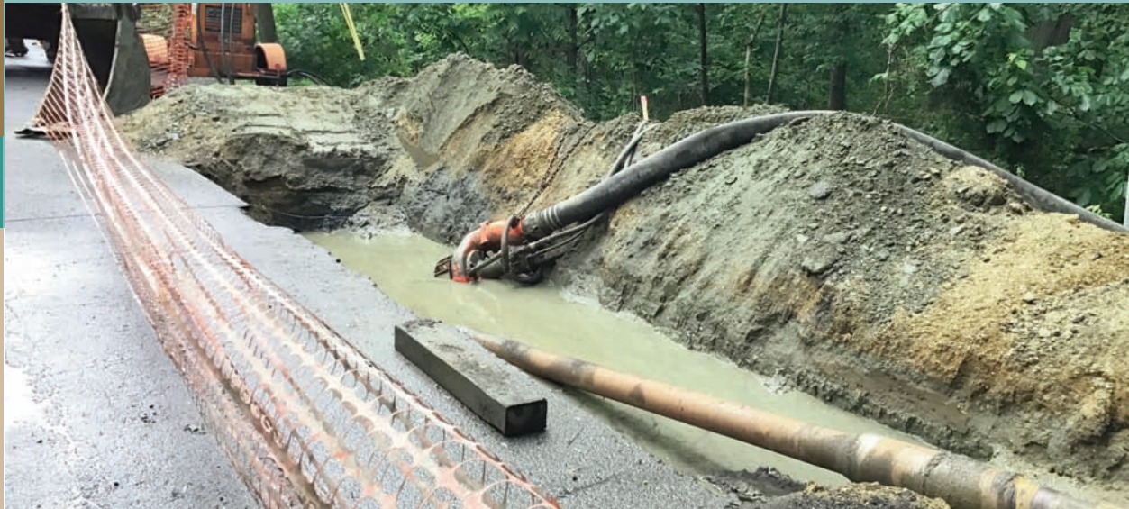
Drilling for New Jersey Natural Gas pipeline in Upper Freehold Township in June. Photo credit: Patti Caruso.
