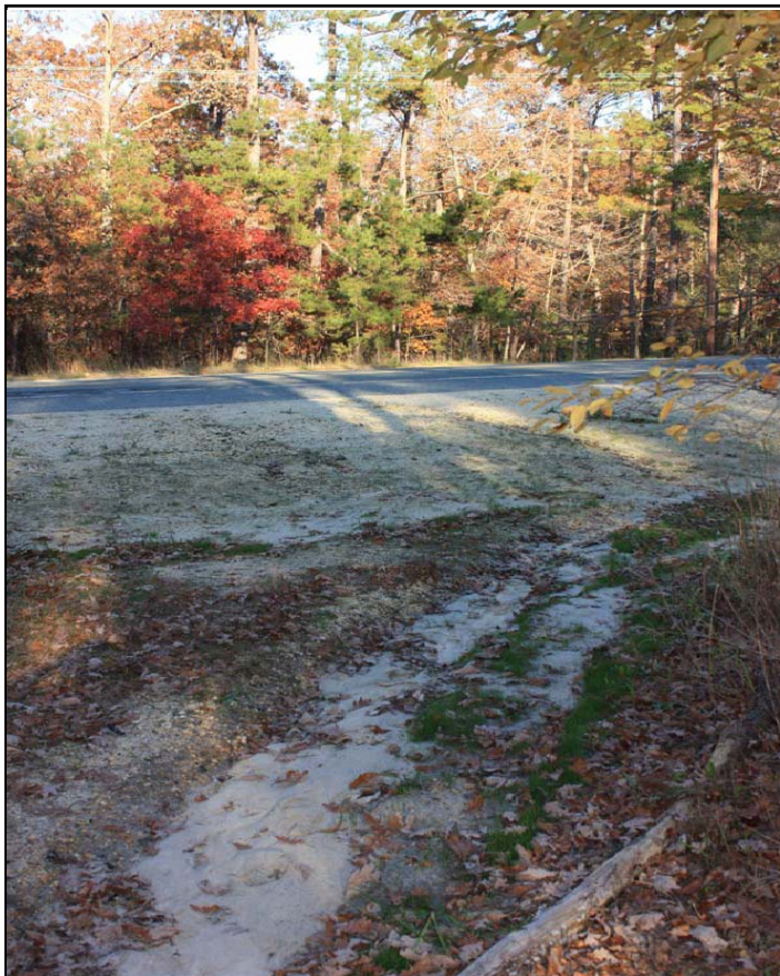
Roadside erosion that intruded 240 feet into the Preservation Area of the Pinelands after a small gasline was placed along Rt. 72 to service the New Lisbon Development Center.
